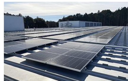
The solar system at Shiroi Data Center Campus
